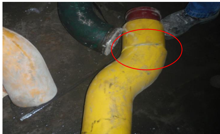
Photograph of a CDD which has been separated at the pull linkage
